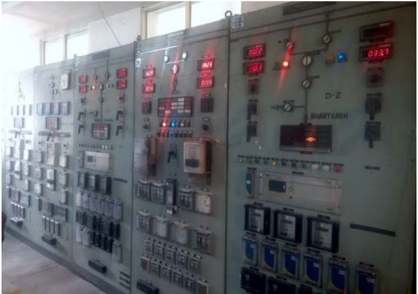
The Burnt panels of 132 KV Substation were replaced by new panels and Asron-Ropar Line was energized in time and 132 KV supply was restored in only 4 hours
